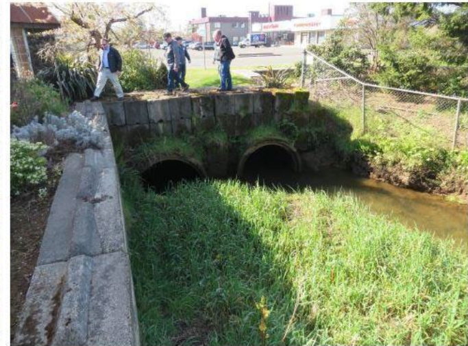
FRY CREEK - CULVERT CONSTRICTIONS
