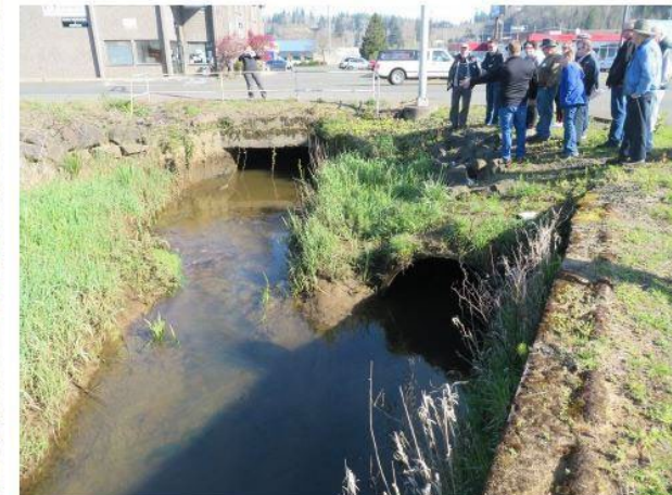
FRY CREEK - CULVERT CONSTRICTIONS
