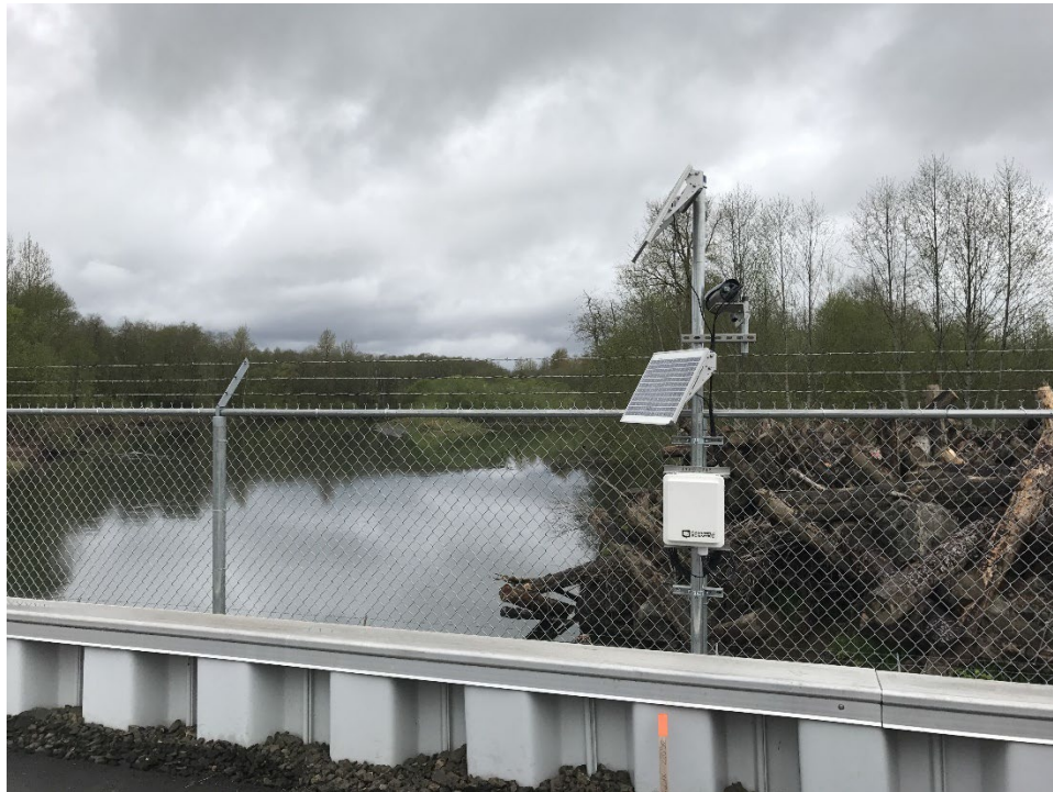
Figure 3.2. Webcam installed at the Wynoochee River at Montesano WWTP.
