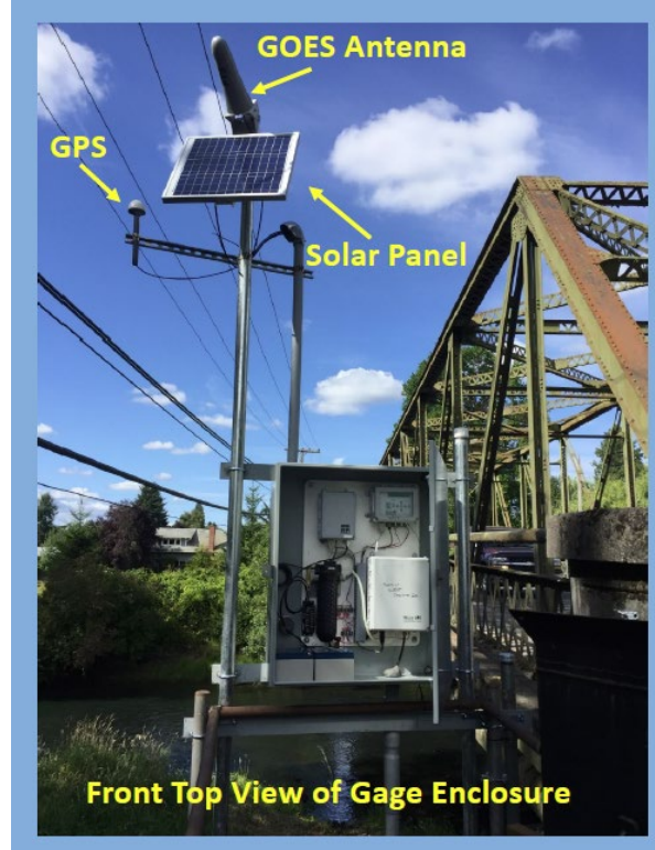
Figure 2.1. Skookumchuck River at Centralia upgraded gage house with bubbler sensor and satellite telemetry.
