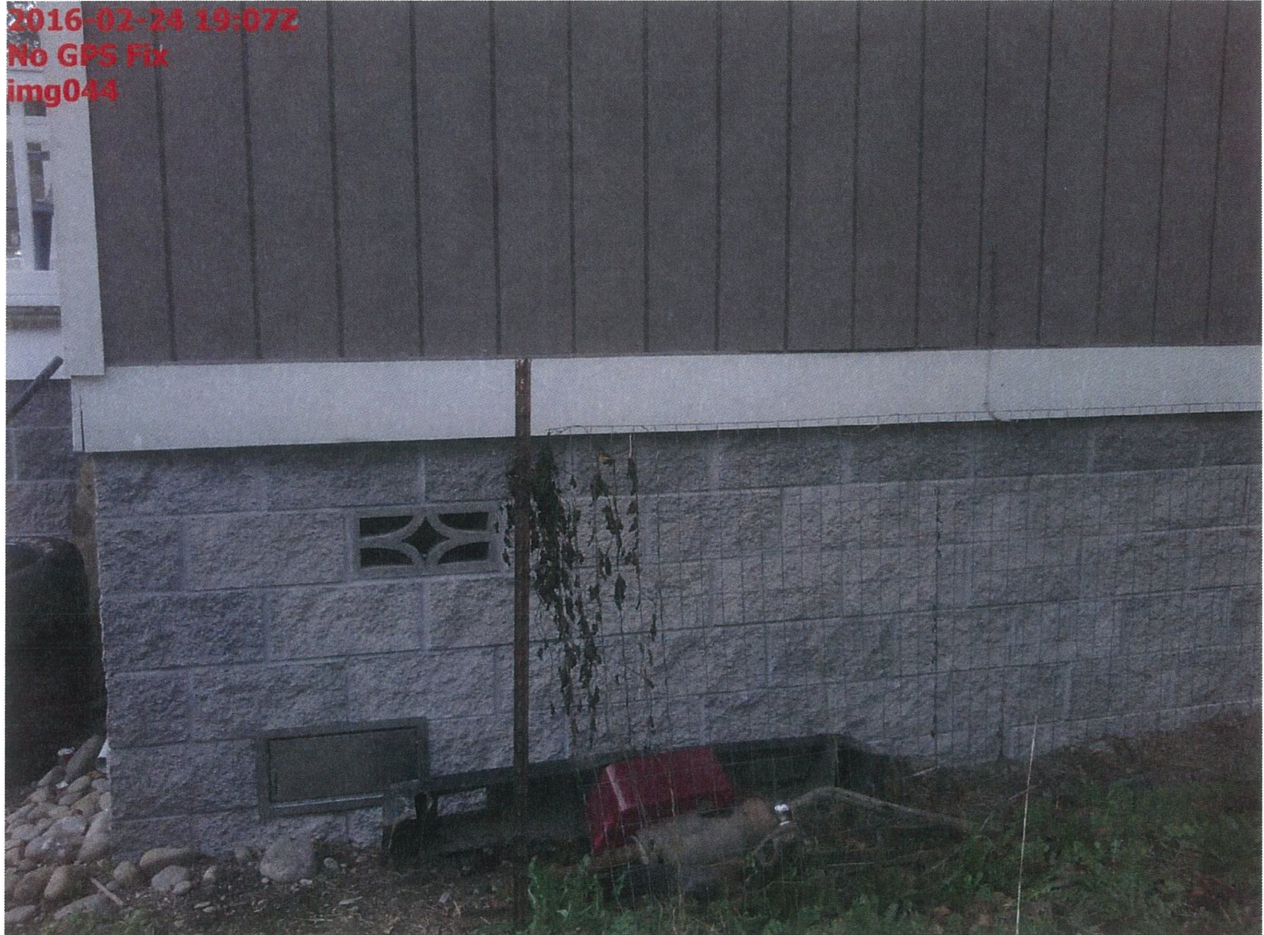
East (front-right) corner of house. Front of house faces southeast to N Market St.
