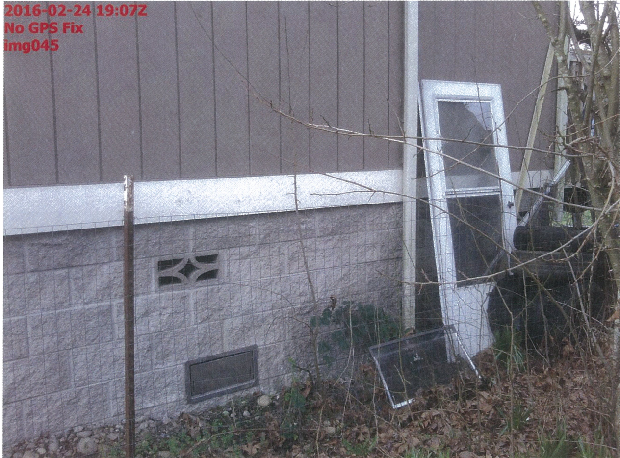
North (back-right) corner of house. Front of house faces southeast to N Market St.
