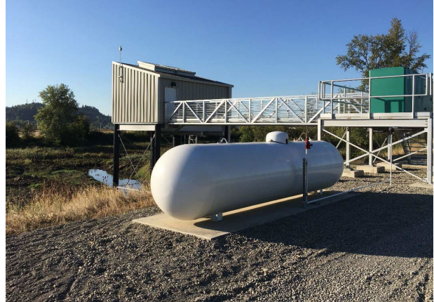
Figure 2 – After, today's pump station
