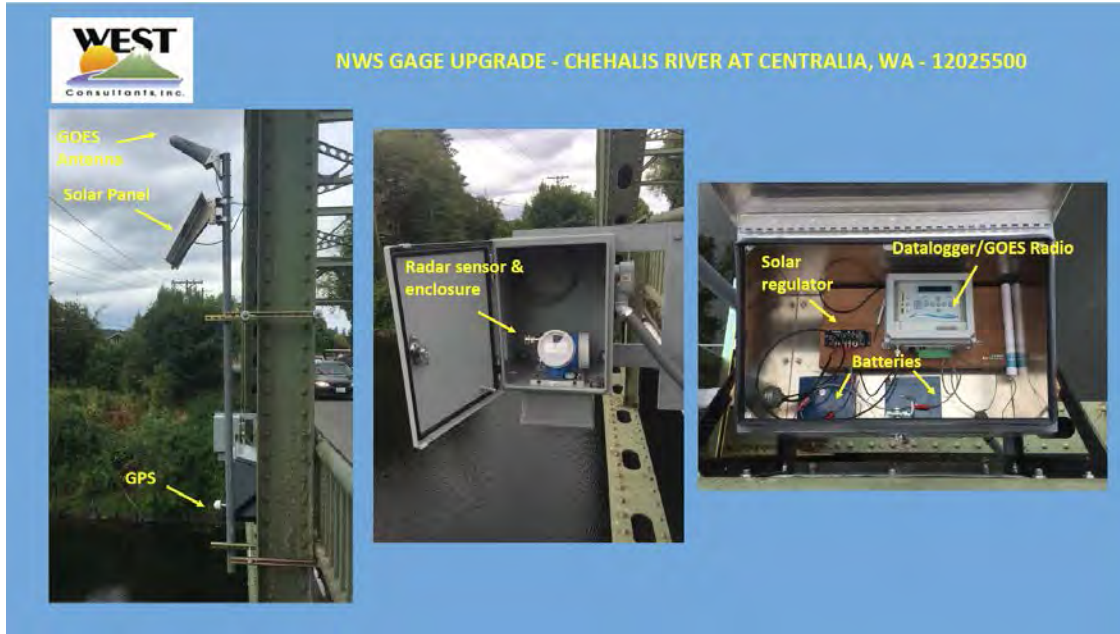
Figure 5-2. NWS Gage Upgrade Chehalis River at Centralia, WA
