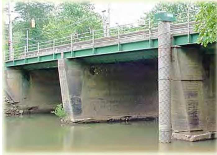
Figure C-10. USGS stilling Well Attached to a Bridge in a Stream
