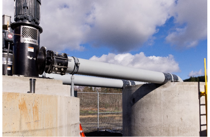
Ramer Street Pump Station (pic 2):
