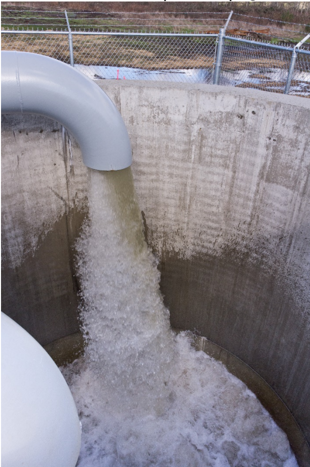
Ramer Street Pump Station (pic 3):
