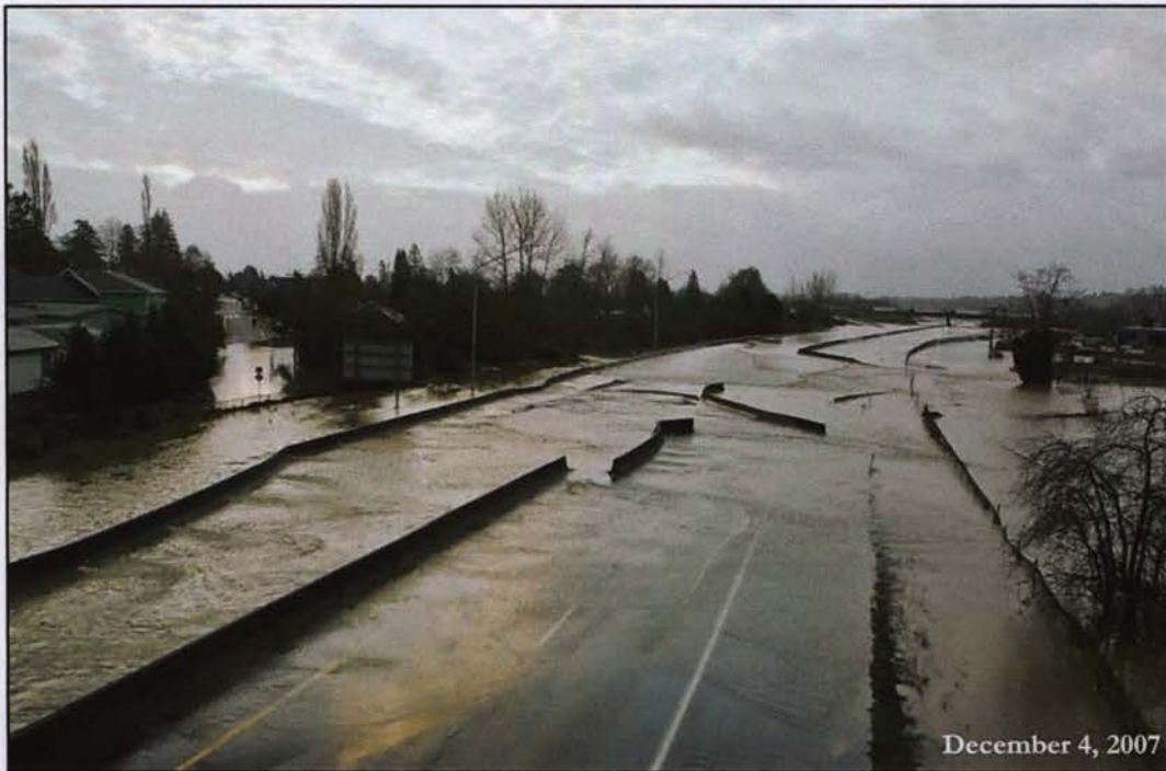
Figure 4. Barrier breach during December 2007 flood event.
