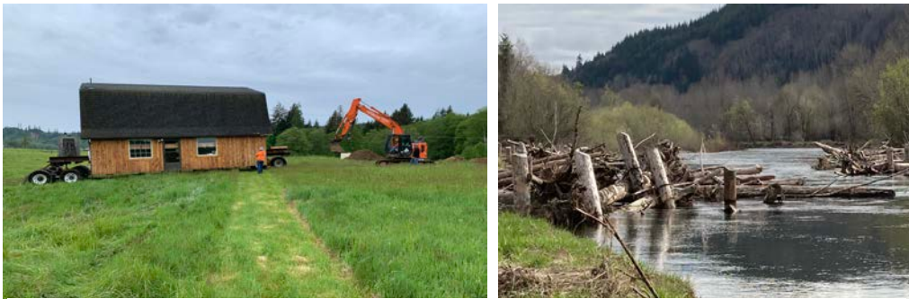
The house relocation (above, left) was a key element in the collaboration between a landowner and project partners. Engineered log jams (above, right) are an important habitat component for the Wynoochee River Restoration Project.
