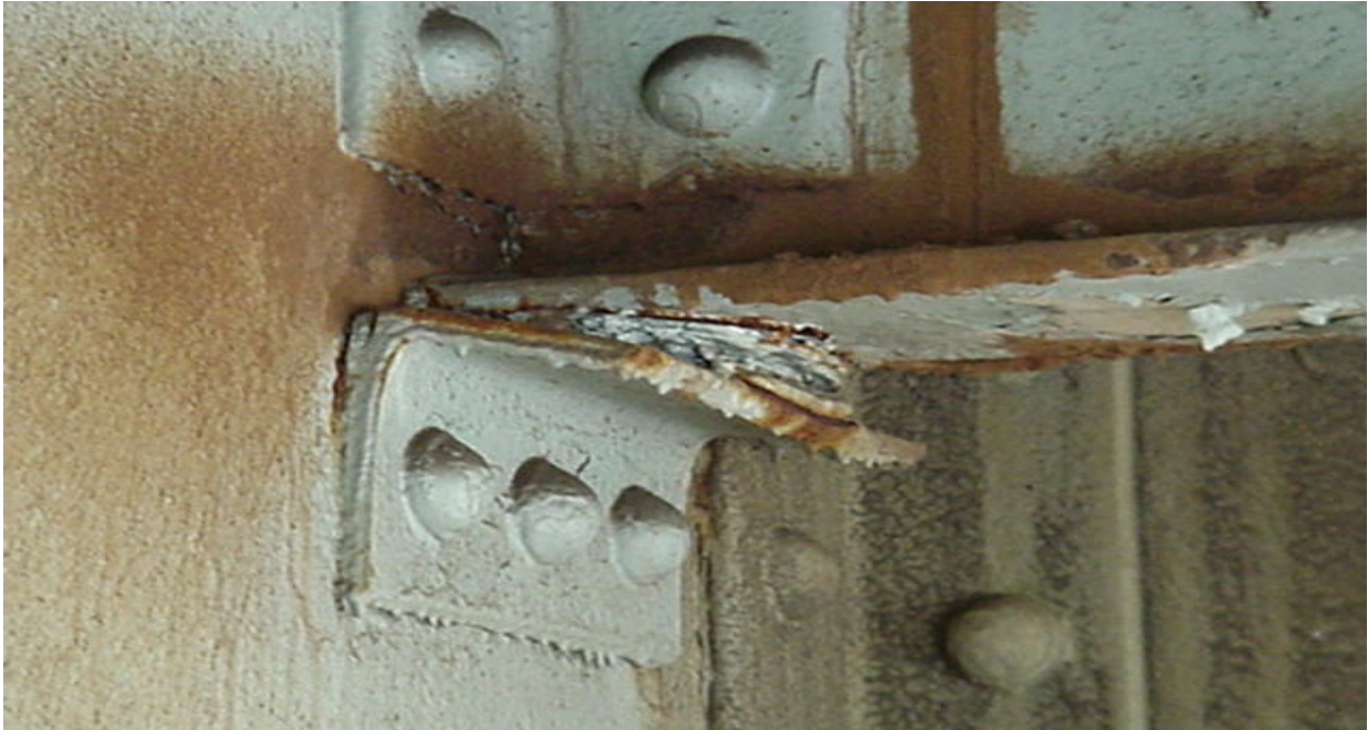
Puyallup River Bridge – Typical rust in beams
