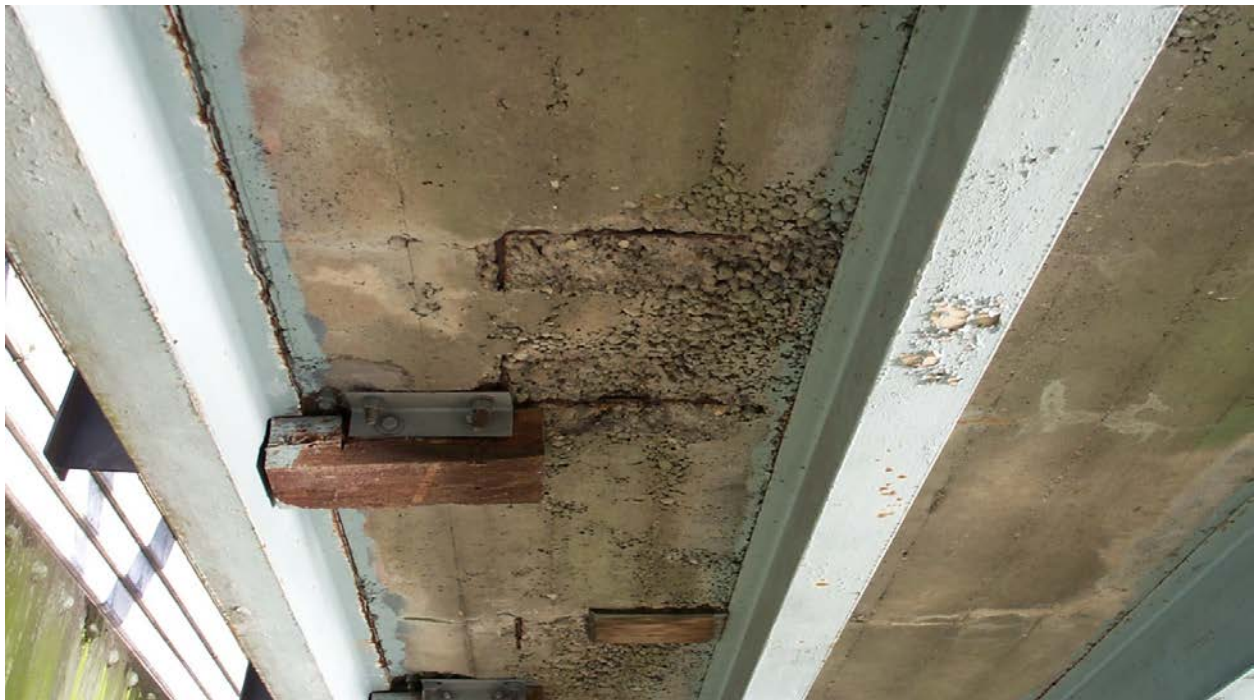
Existing Puyallup River Bridge – Concrete Spalling
