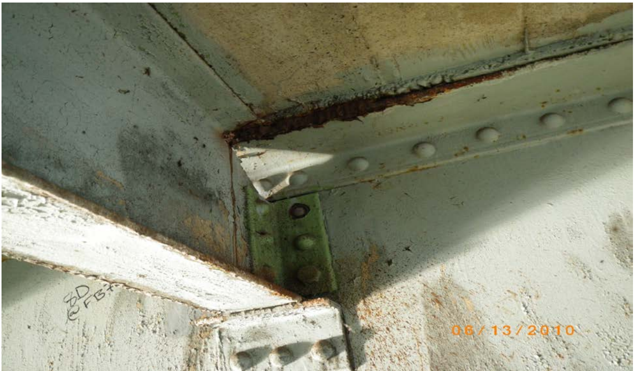
Puyallup River Bridge – Typical broken Rivet
