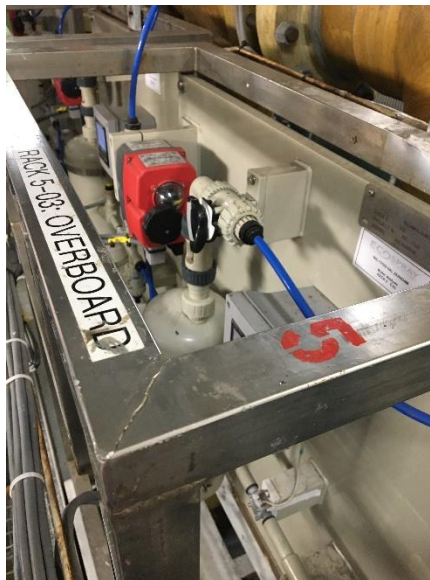
Monitoring rack; ZAANDAM 7-30-18 Jankowiak
