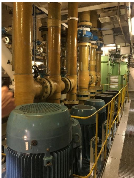
Water feed pumps and mixing/dilution pumps; ZAANDAM 7-30-18 Jankowiak
