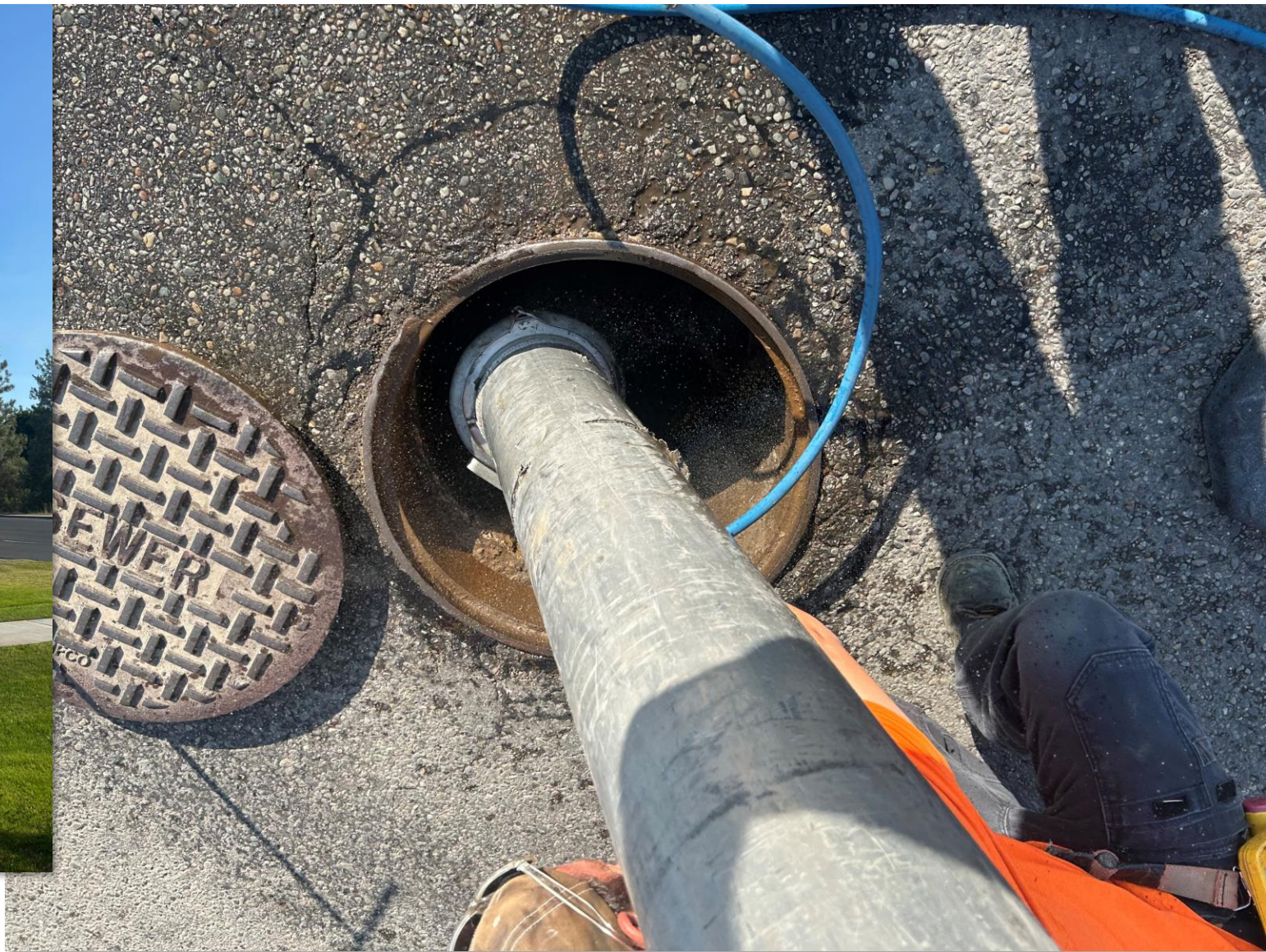
ERTS #724213 Kelowna Corp/Chevron Fuel Station Diesel Spill
