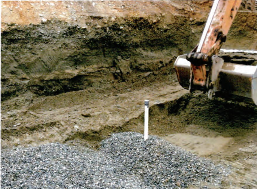
Picture 2: [Looking NW] BC-3 installation of 2" PVC for piezometer in pit drain area. Subgrade at northern end of infiltration region is a sand rather than a gravel.
