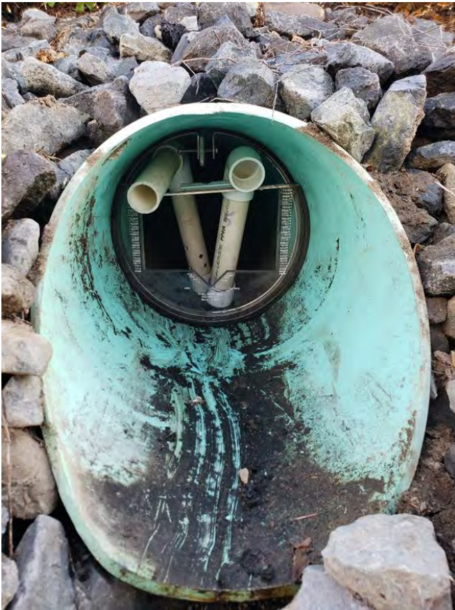
Figure 2. Inflow Monitoring in the Inlet Pipe at TWH_IN1
