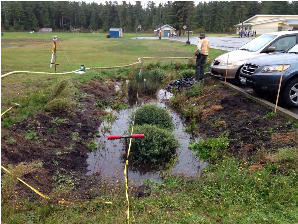
Cell TBM during infiltration testing, looking southeast, after about 1.5 hours of inflow.
