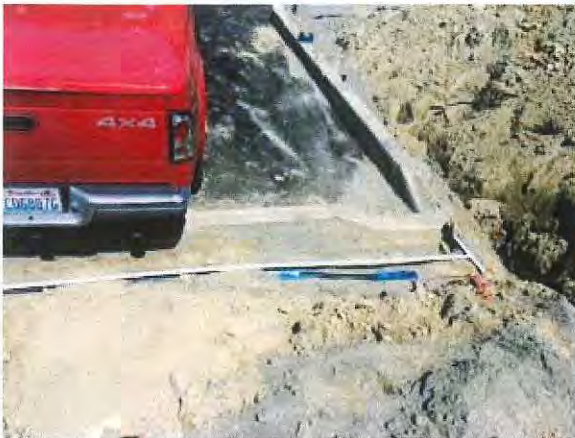
Entry point cell 6 not complete
