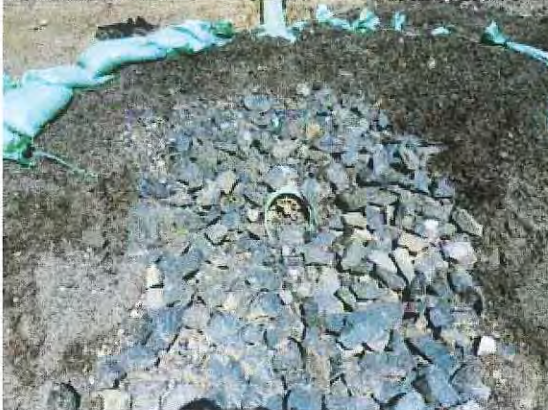
Plugged area drain to cell # 9
