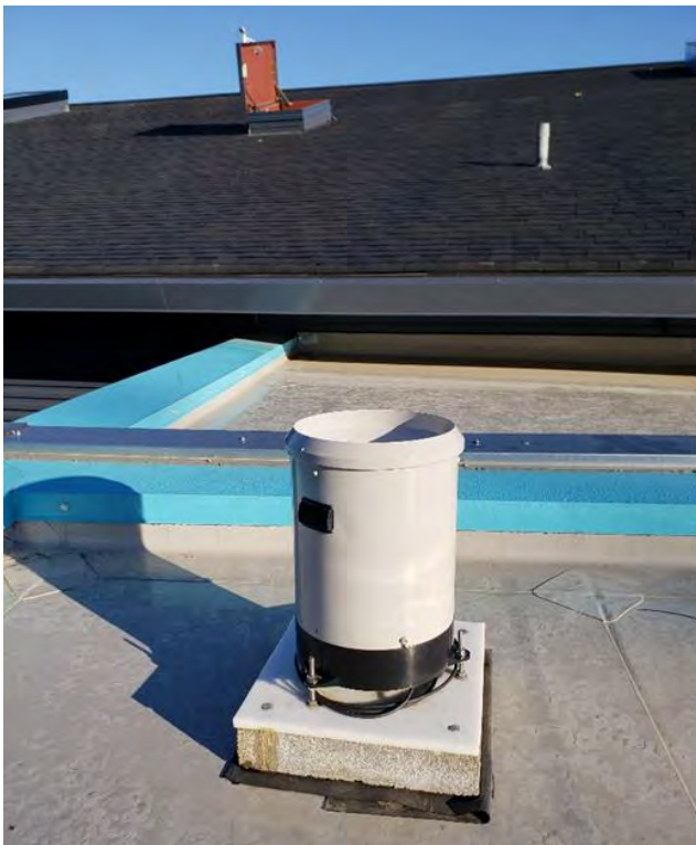
Figure 1. Rain Gauge Installed on Salem Woods Elementary School Roof (SSW)
