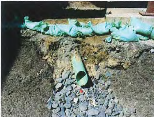
Erosion at cell # 9
