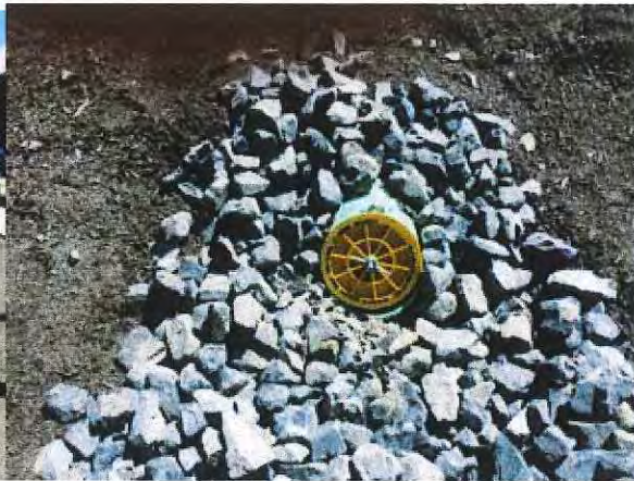
Plugged catch basin to cell # 5
