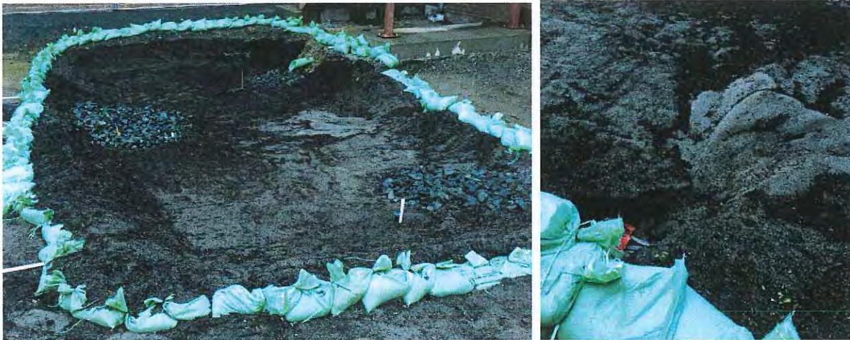
Left: BR9 showing native material on the bioretention mix surface. Right: Close up of a blow out and the resultant plume/delta on the bioretention mix.
