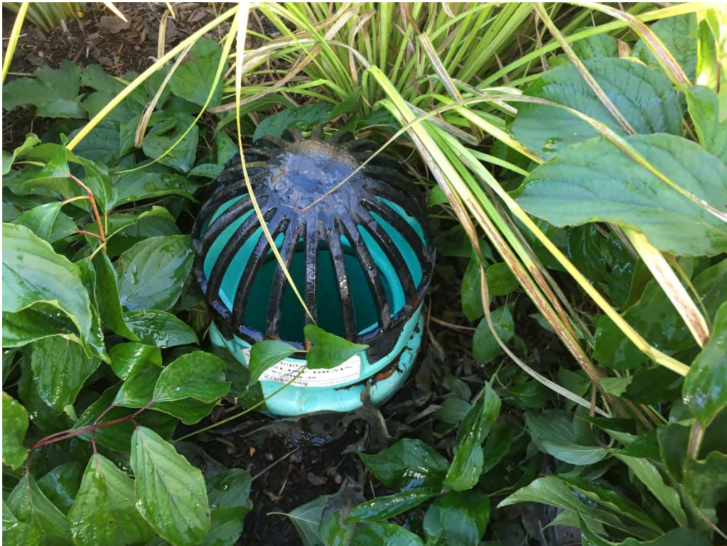
Above photo: M1C primary inlet. Lower Photo: close up of overflow structure.
