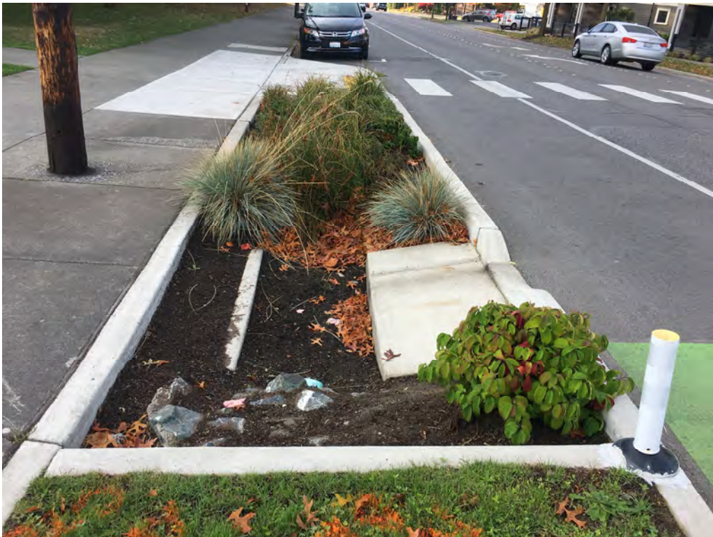
Cell BCK overview, curbcut inlet shown
