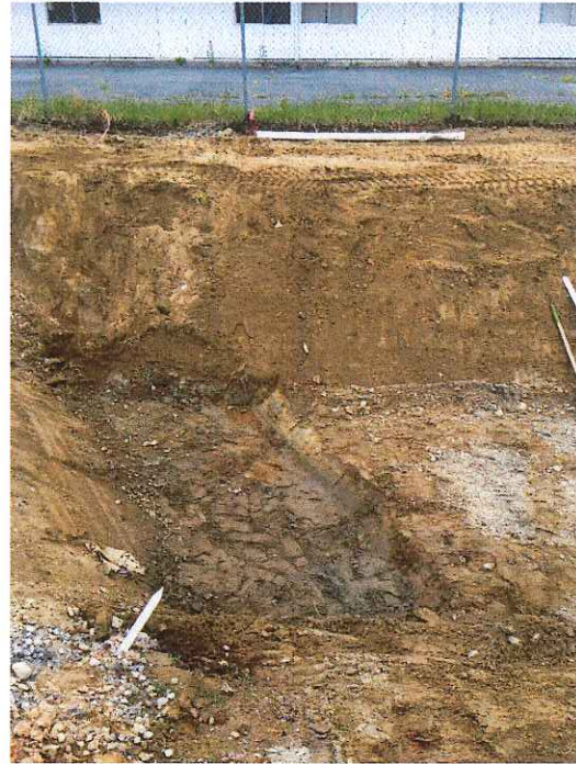
Photo 2 (right): Area excavated an additional ~0.5' at the north end of the cell.
