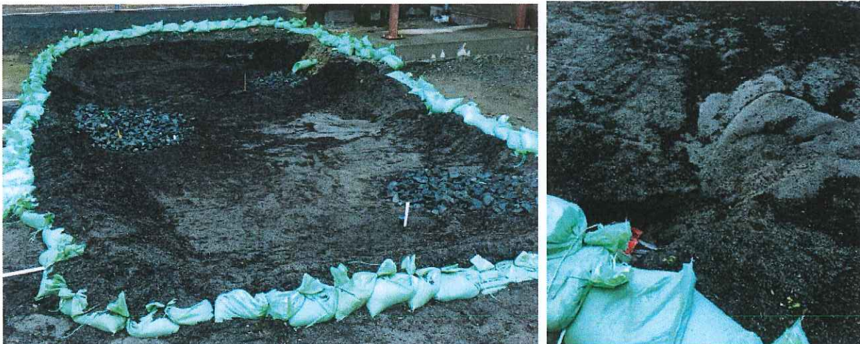
Left: BR9 showing native material on the bioretention mix surface. Right: Close up of a blow out and the resultant plume/delta on the bioretention mix.
