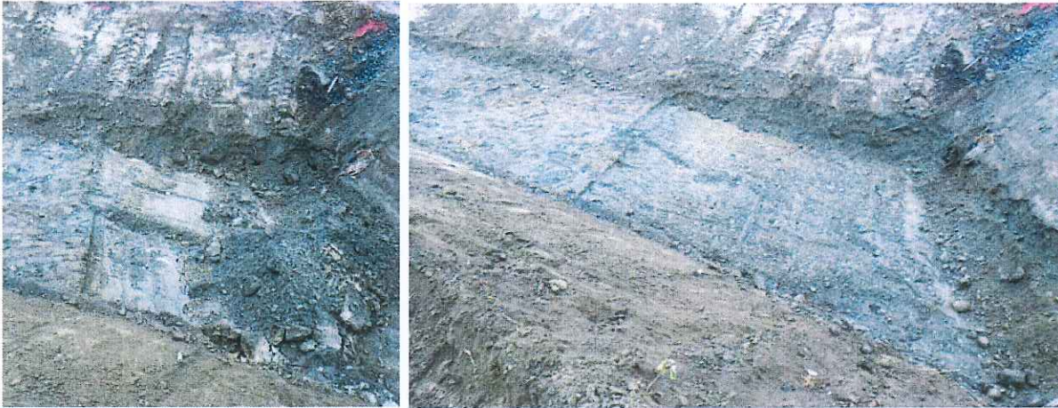
Left: BR6 viewing west; removal of silty sediments under way. Right: finished product after silty sediment removal.
