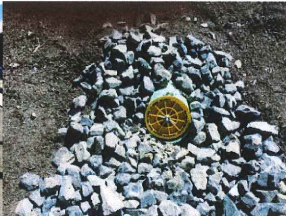
Plugged catch basin to cell # 5
