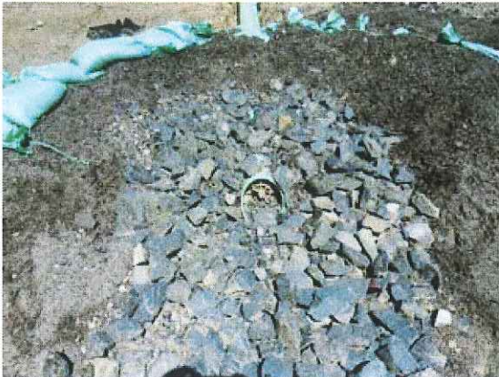
Plugged area drain to cell # 9
