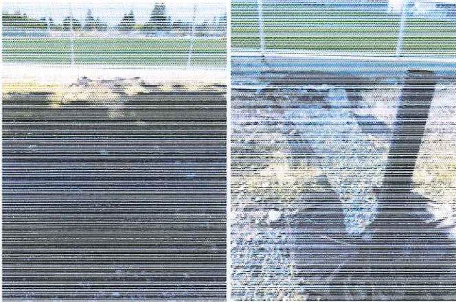
SW ballfield infiltration trench NW ballfield infiltration trench to be covered today
