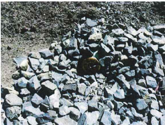
Area drain plugged to cell # 10
