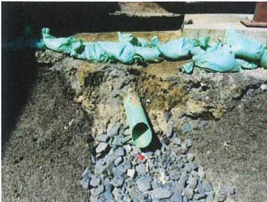
Erosion at cell # 9
