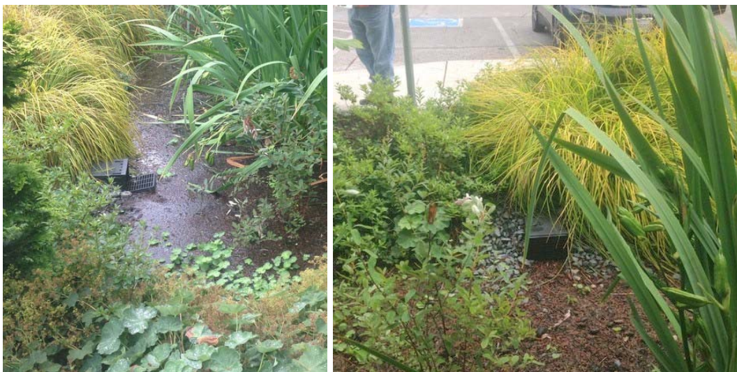
Photo 1. Cell MCCA2, 8-inch “overflow” yard drain grate, oriented sideways instead of vertical.
