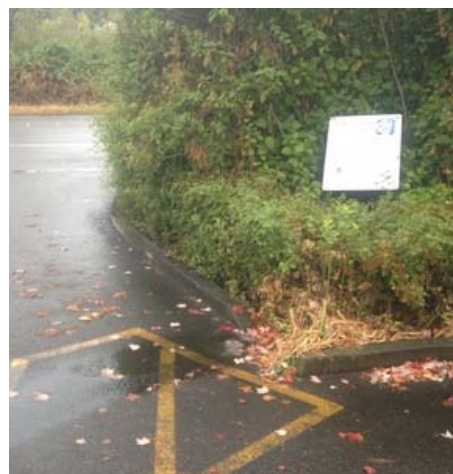
Photo 1. Cell BDP, southeastern inlet clogged with leaves. Some water bypass toward Electric Avenue. 9/2/16.
