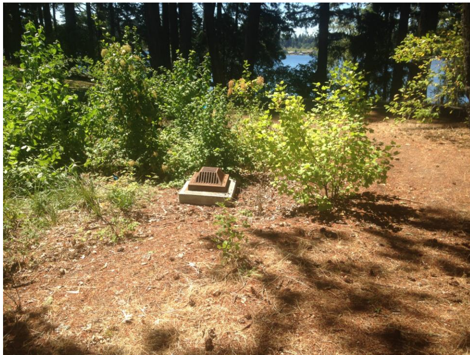
Cell SLP"J" overflow structure
