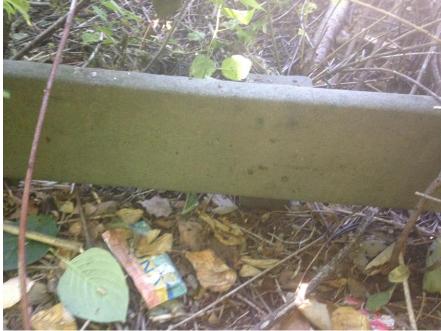
Gap under weir board in Cell BDP
