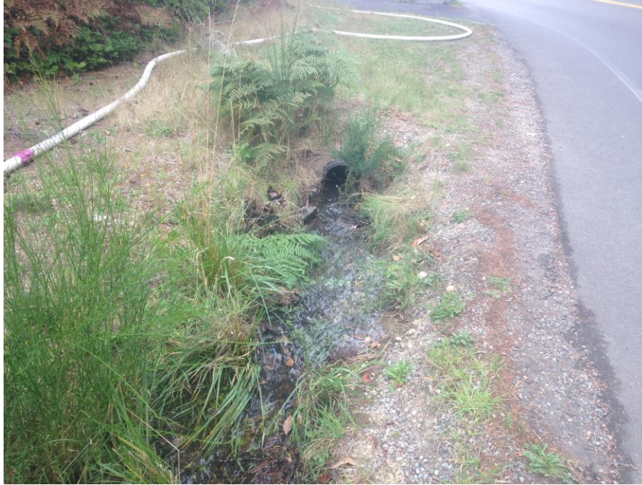
Discharge from overflow pipe during infiltration testing
