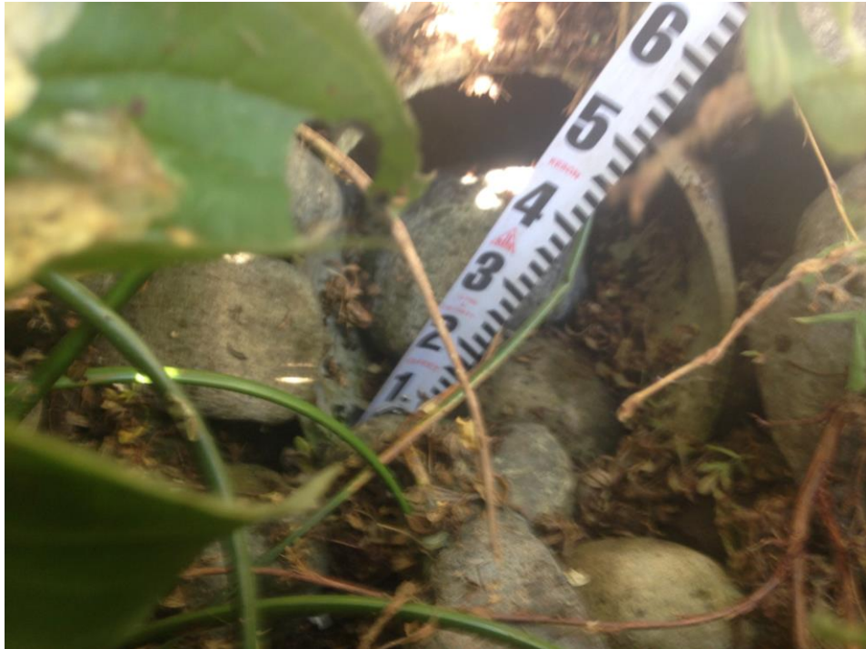
An inflow pipe to ORLA 2-B.
