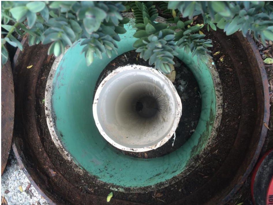
Cell B145 pre-existing observation port
