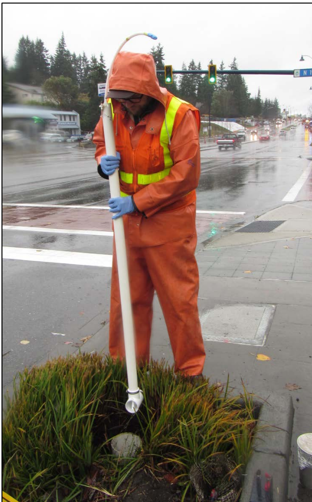
Figure C-4. BPB1 outlet sampling, PVC pole holds tubing along the bottom of underdrain (December 8, 2015).
