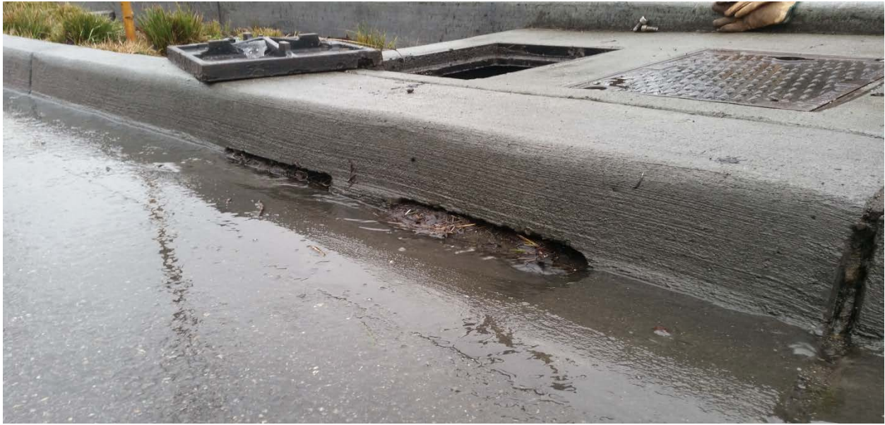
Figure J-1. Debris blocking curb cuts at BPB1 inlet (January 21, 2016).
