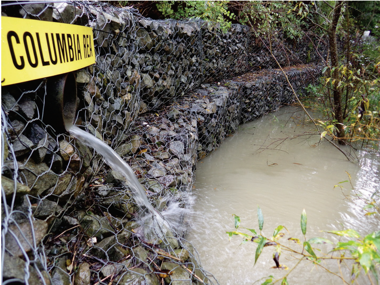
Figure 2. Turbid discharge from a minor pipe to old CDSTW on October 20, 2016.
