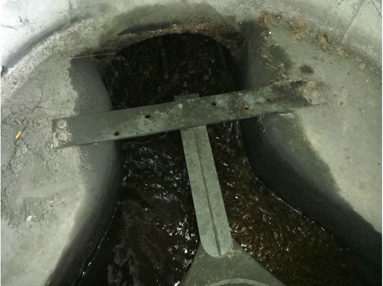
Figure 1-A. Source vault for I-5 stormwater, flow in photo is from top to bottom.
