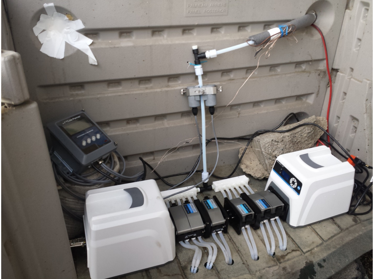
Figure 6-A. Stormwater dosing pumps, distribution manifold, and flow totalizer.
