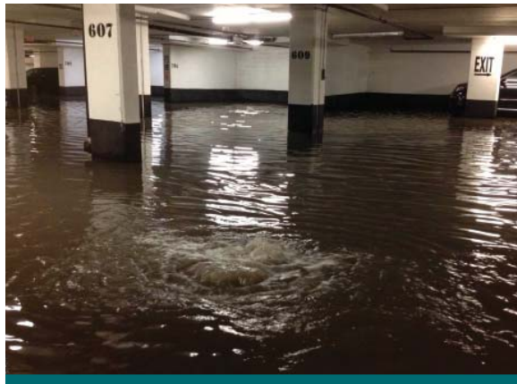
Figure 1.1.5: This photograph shows an underground parking structure during an extreme event. Could this be your property? (Source: CVC)
