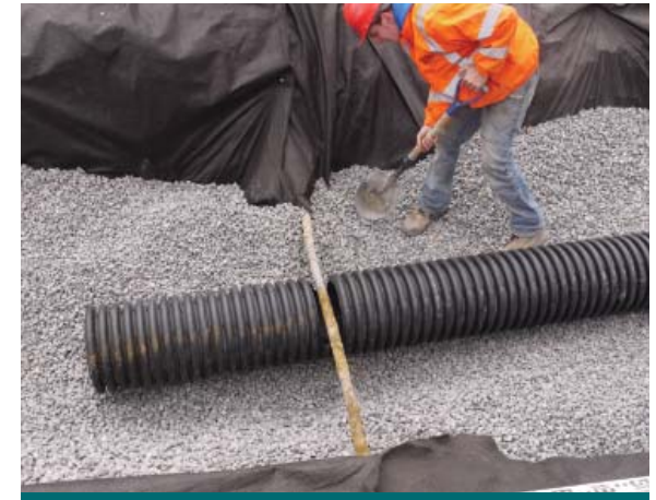
Figure 9.4.2: The construction team cuts a notch a perforated pipe to accommodate a gas line. (Source: Aquafor Beech)
