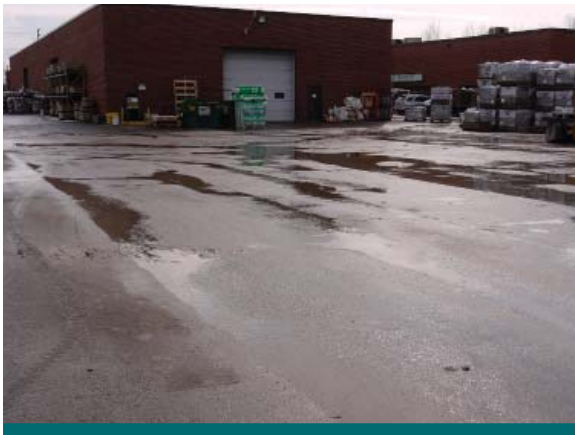
Figure 4.1.4: Improper surface grading can reduce a site's drainage capabilities. At this site, most rainfall causes significant ponding and interferes with day-to-day operations. (Source: CVC)
