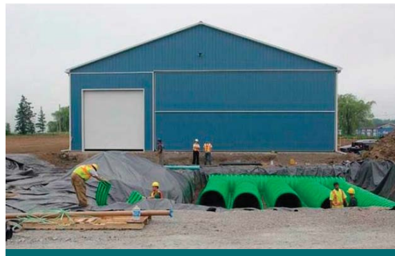
Figure 2.7.2: In this design, rainwater is collected in a modular subsurface system and used for emergency fire suppression. (Source: Aquafor Beech)
