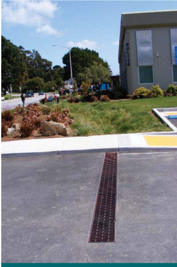
Figure 6.4.7: Grated strip drains ensure onsite control at parking lot entrances. (Source: Aquafor Beech)
