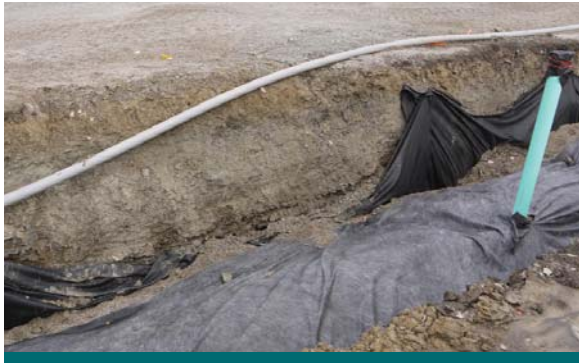
Figure 9.6.1: Infiltration areas are covered with sacrificial strips of geotextile when filled with media to protect them from contamination. Contractors can then clean out debris without affecting the infiltration area. (Source: CVC)
