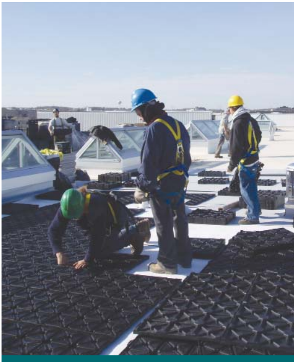
Figure 9.5.1: Mechanical and structural components may interfere with installation on flat roofs. Here contractors work around ventilation components and skylights. (Source: CVC)
