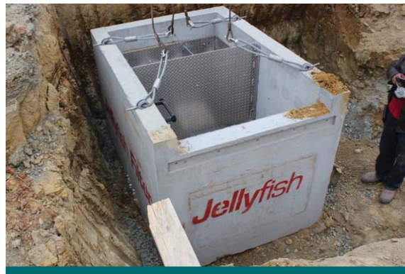
Figure 2.9.5: To maximize treatment and water balance benefits, proprietary stormwater treatment devices can be installed upstream of LID practices. (Source: CVC)
