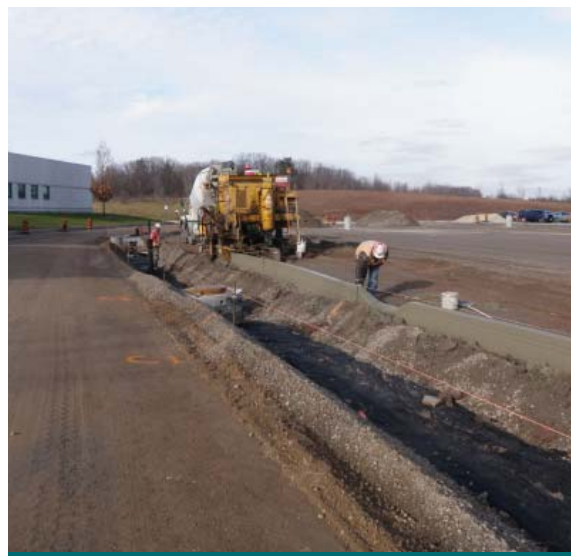
Figure 6.4.25: The bioswale and new curbing being installed at the IMAX Project. (Source: Aquafor Beech)
