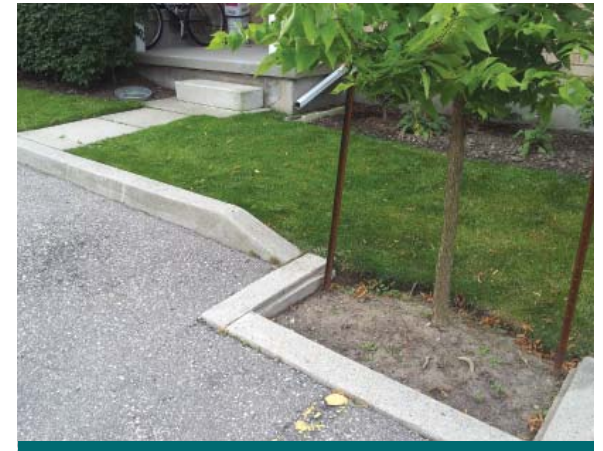
Figure 4.8.3: This parking area could be retrofitted with permeable pavement. The green area on the opposite side of the curb provides a suitable location for a small bioretention planter accepting roof runoff. (Source: Aquafor Beech)
