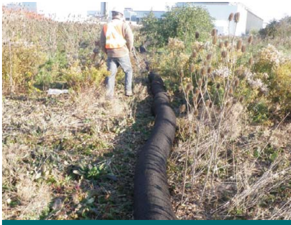
Figure 9.6.2: A filter sock installed at the IMAX Project site as part of the erosion and sedimentation control plan. (Source: Aquafor Beech)
