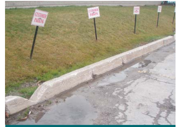
Figure 1.2.7: Storms can create liability issues for business owners. Flooding and the resulting infrastructure damage can harm customers and their property. (Source: CVC)
