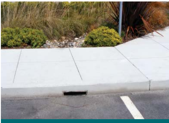
Figure 6.4.4: The covered curb inlet is a common feature of conventional and LID designs. (Source: Aquafor Beech)
