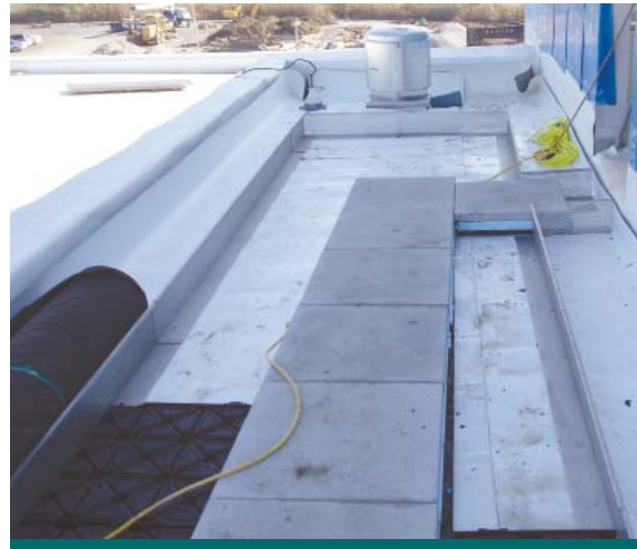
Figure 9.5.2: Contractors installed planks to avoid walking on delicate roofing components. (Source: CVC)
