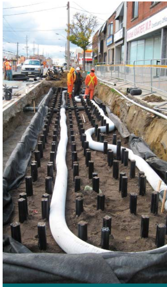
Figure 2.9.3: During installation of a soil support system, significant excavation will be required. Modular units allow for design flexibility, such as this long configuration. (Source: DeepRoot)
