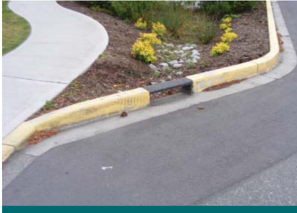
Figure 6.4.10: A cover on a curb cut can provide a barrier that prevents damage from snow removal operations. (Source: Aquafor Beech)
