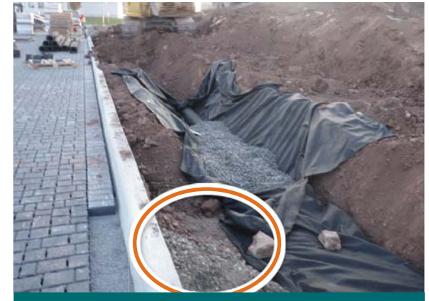
Figure 9.2.3 The granular base of the permeable pavers extends into an adjacent trench constructed for a perforated pipe system installed during the IMAX Project. In the design, the two features were to be hydraulically separated by a clay plug. (Source: Aquafor Beech)
