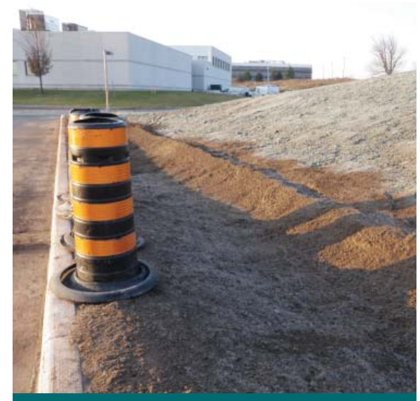
Figure 9.3.2: Approved bioretention soil media is installed at the IMAX Project site. (Source: Aquafor Beech)
