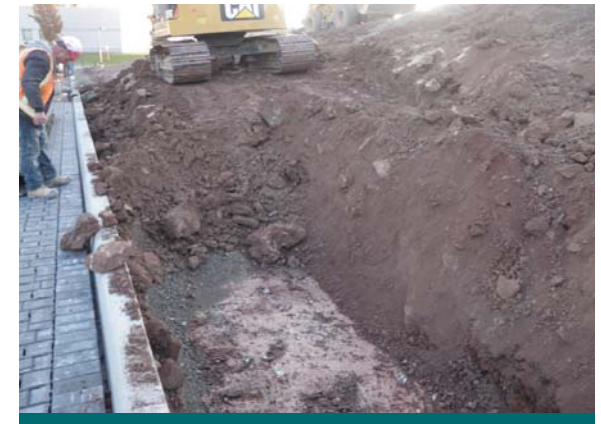
Figure 9.2.4: The granular base has been removed from the perforated pipe area. (Source: Aquafor Beech)
