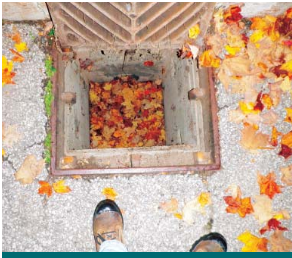
Figure 6.4.19: Coarse materials like leaf debris will collect in catch basins and obstruct flow. They require monitoring and regular maintenance. (Source: Aquafor Beech)
