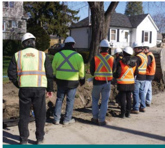
Figure 9.2.1: Contractors, construction supervisors, designers, project managers, site inspectors, and surveyors meet at weekly site meetings to discuss issues and develop solutions. (Source: CVC)
