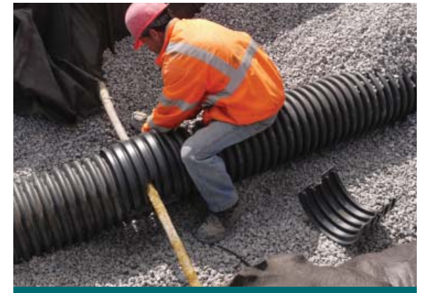
Figure 9.4.3: The team adds a section of perforated pipe to the top of the notch to prevent granular material from creating a blockage in the pipe. (Source: Aquafor Beech)
