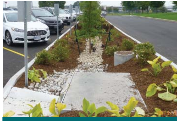
Figure 2.3.2: This parking lot bioretention area treats runoff from a conventional asphalt parking lot. It incorporates additional proprietary stormwater treatment devices within the bioretention to provide even greater water quality treatment. (Source: CVC)
