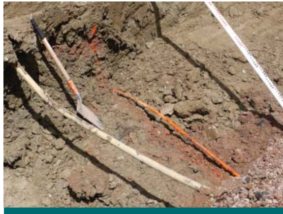
Figure 4.1.2: Utilities are major barrier to construction. The pipes pictured above were not listed in the background information and caused construction delays as excavation had to work around them. (Source: CVC)
