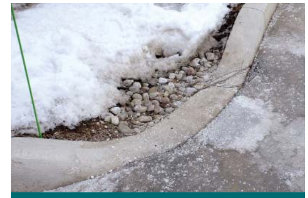
Figure 4.9.3: This curb cut had to be cleared to allow water to flow into the practice. (Source: CVC)
