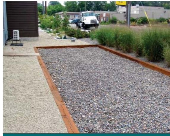
Figure 2.5.1: Redirecting roof drainage to a soakaway pit is a simple but effective way of reducing the volume of water from your site. For roof runoff, pre-treatment is not required. (Source: Aquafor Beech)
