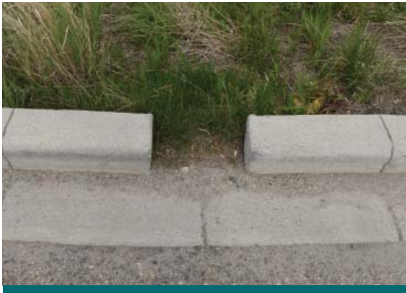
Figure 6.4.1: This notched curb cut at the City of Calgary's City Hall provides flow to a bioretention area from a parking area. More notches may be required to match the inlet capacity of a curb cut. (Source: Aquafor Beech)
