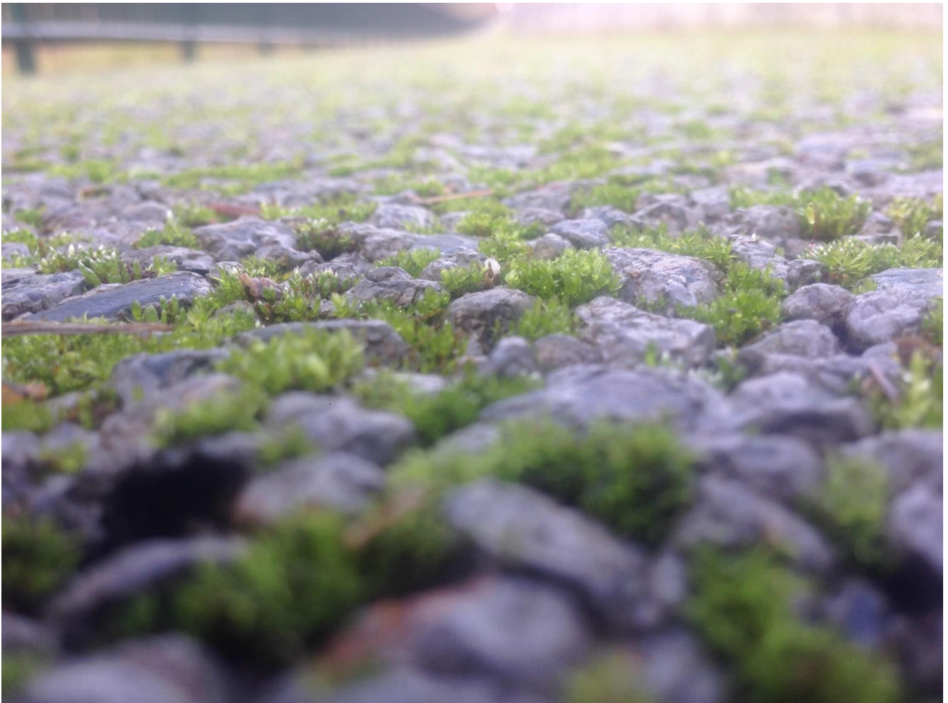
Figure 5. Closeup of moss growing on permeable pavement sidewalk.
