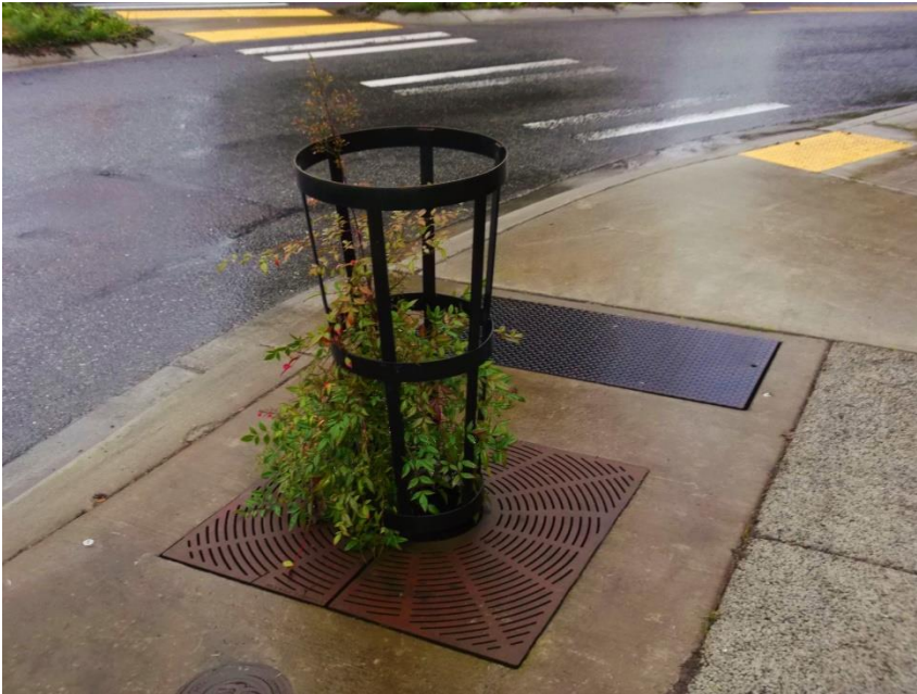
Figure 7. Filterra® system installed along high-traffic roadway.
