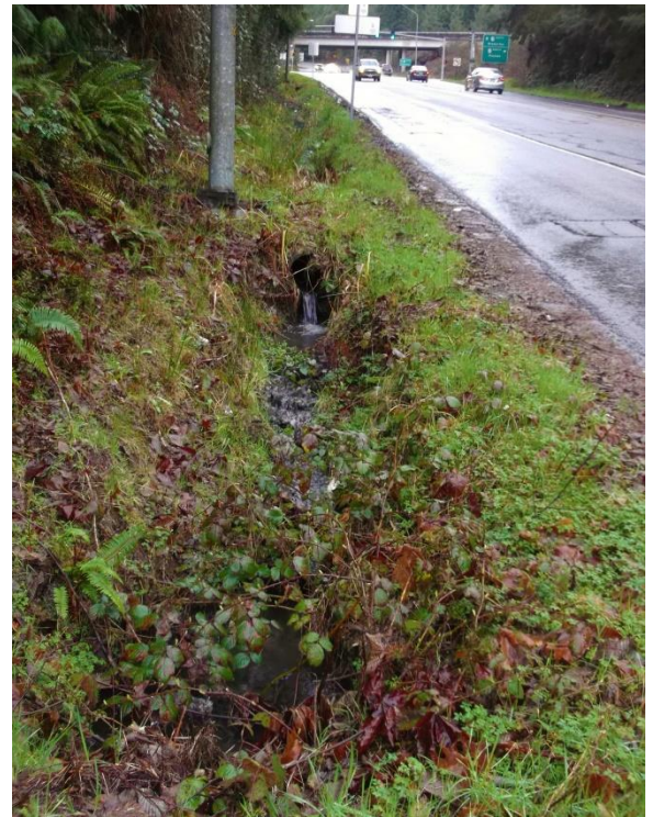
Figure 8. Roadside ditch during a rain event.
