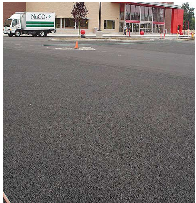
In an asphalt parking lot in Snohomish County Washington, pervious asphalt is used in the parking stalls (foreground) and smoother more impervious asphalt is used in the drive aisles (top of photo near cone).
