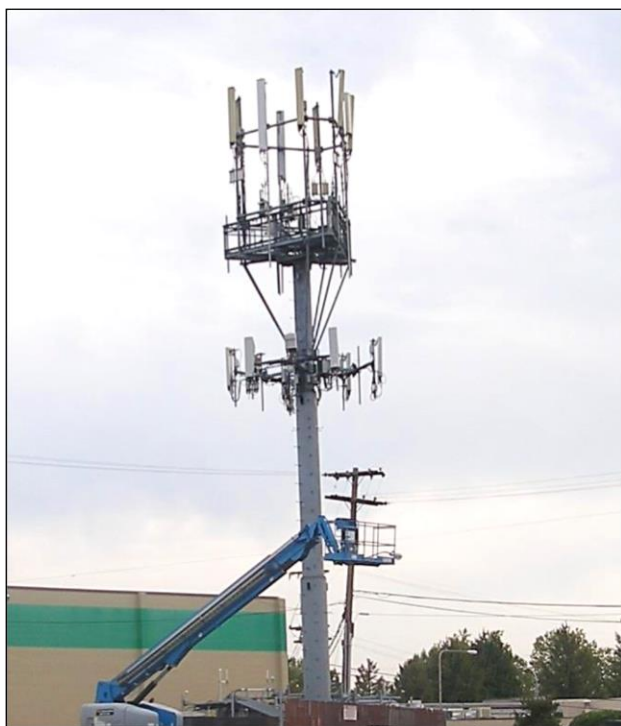
Telecommunications Facility, Credit: City of Renton
