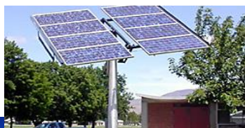
Pioneer Middle School Solar Panels
